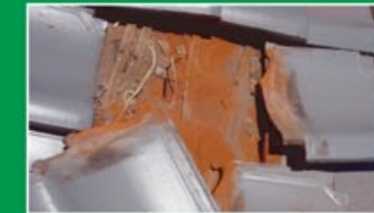
Example of salt damaged roof.
